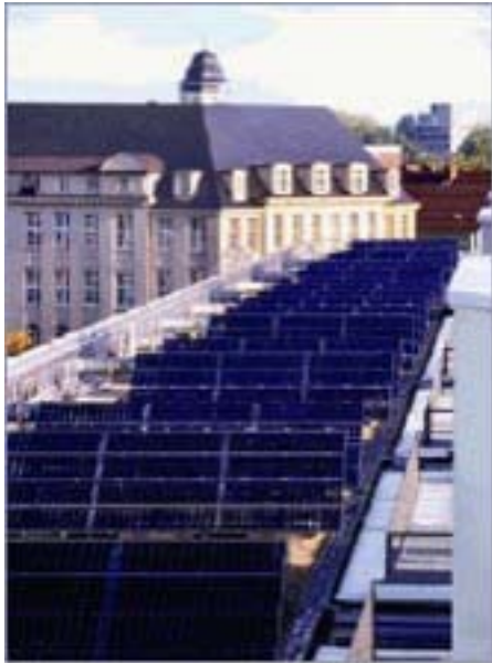
...complete with photovoltaic panels on the roof
