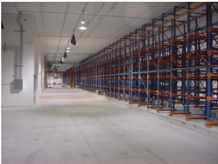
Inside the “battery store” at Golden Valley, November 2002. (Photograph by SAFT)
