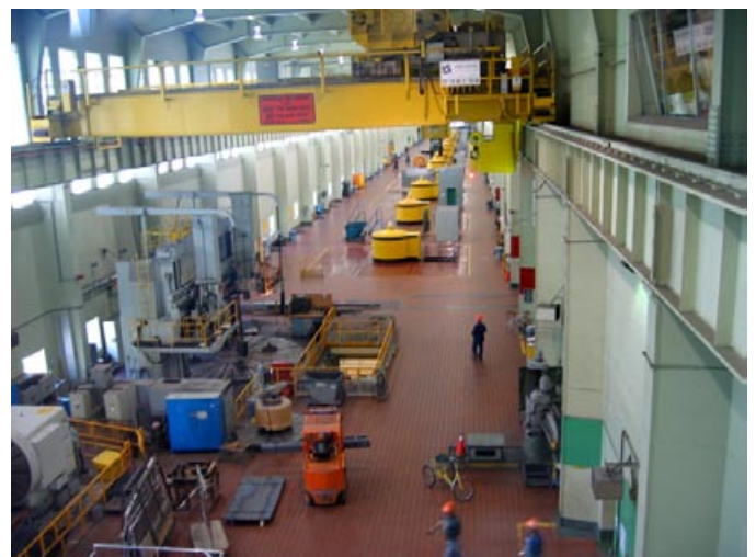
The turbine hall of Ontario Power Generation's Niagara Falls Generating Station.
