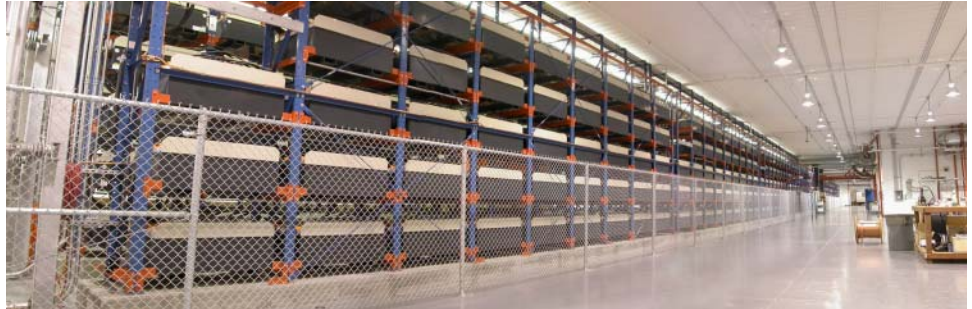
A panoramic view of the battery array. Photo courtesy Saft.
