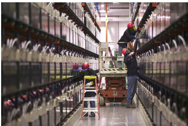
Technicians do a final check on the Golden Valley BESS. Photo courtesy Saft.
