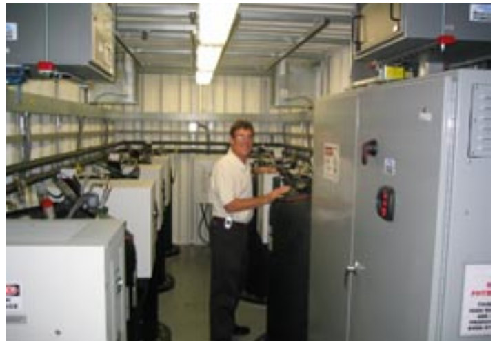
Beacon’s Project Director, Jim Arsenault, inside the flywheel system container.
