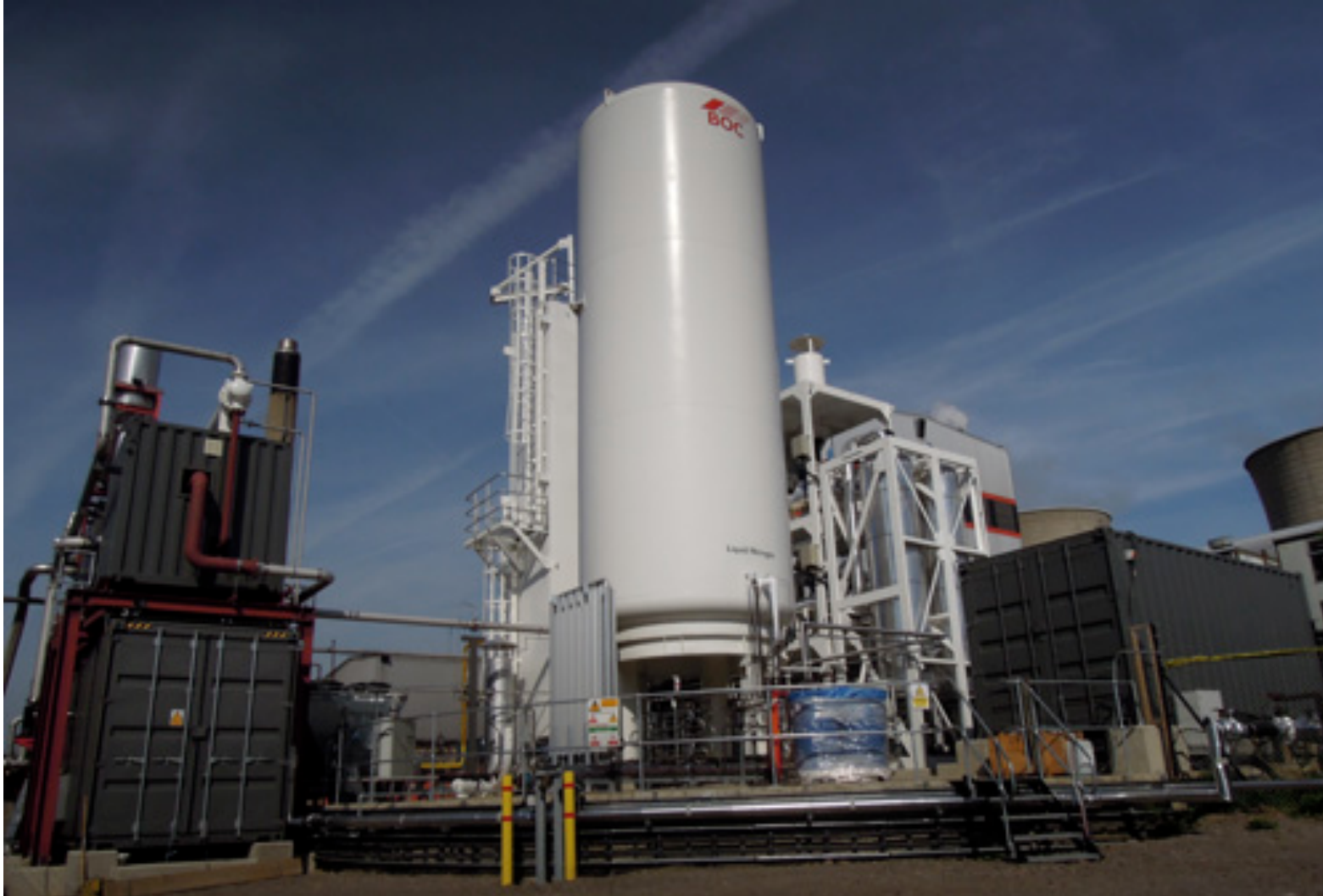
Highview's 300kW/2.5MWh CES plant at SSE's Slough Heat and Power plant, UK. The project has been supported by the UK Govt's Dept. of Energy and Climate Change (DECC).
